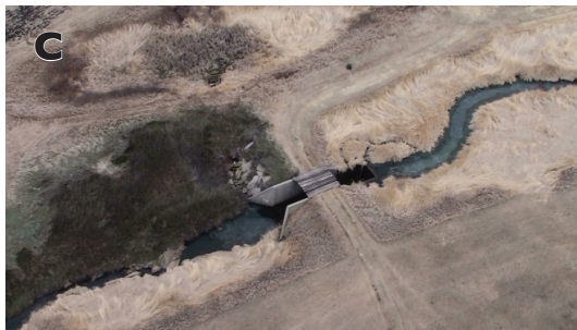
Stage 5. The channel upstream of the grade control structure appears to be relatively stable.
