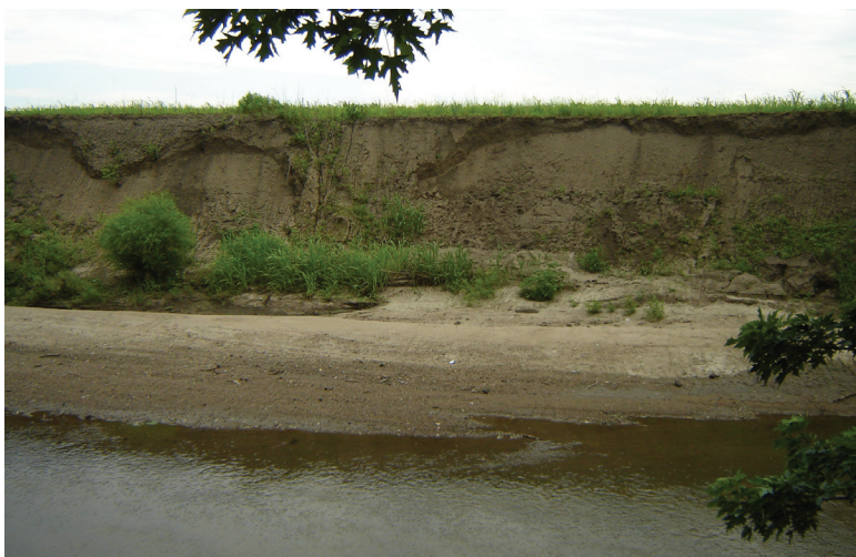
Photo 1. An example of an “area in need of establishment”. These areas, which lack woody riparian vegetation, are expected to generate the highest amount of downstream sediment delivery, in comparison to the other two condition classes. The “establishment” condition class was most prevalent in the Centralia watershed.
